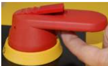
Fig.66: Safety clip on the circuit breaker
